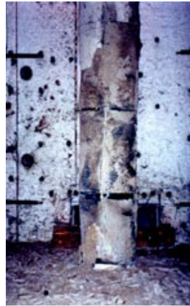
Columns with Tyfo® Composite - still operational after 5 hours of ASTM E119 testing
